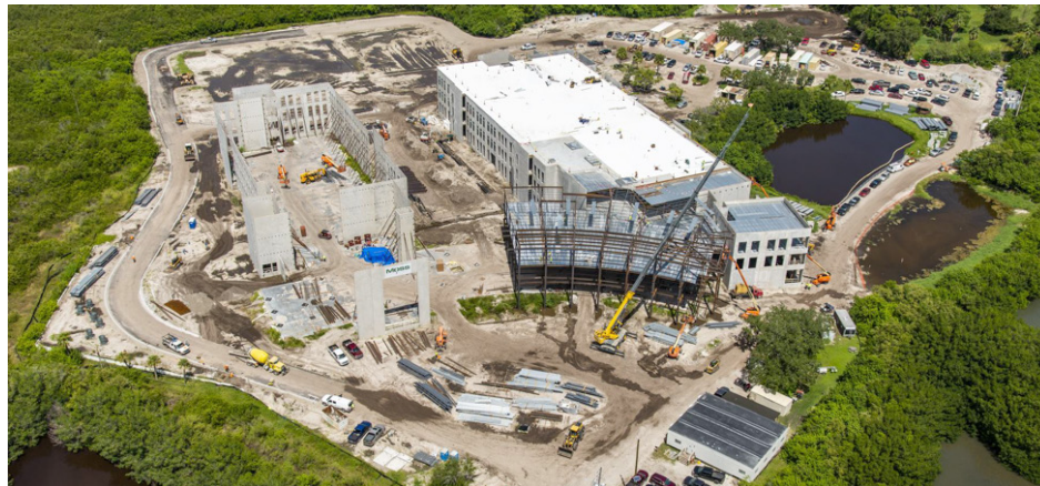
Here is an aerial view from the south side of the construction site taken last month. PRINTED WITH PERMISSION FROM D. ALFONSO
