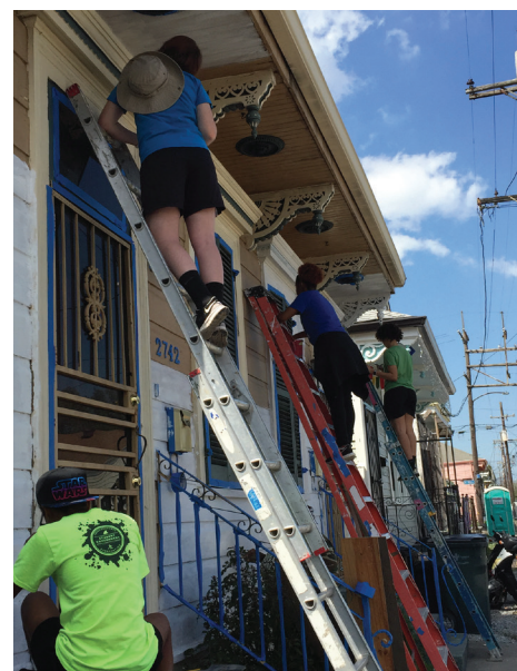
PRINTED WITH PERMISSION FROM M. KNOWLES 2016 SAS spring break trip participants help repair a house.
