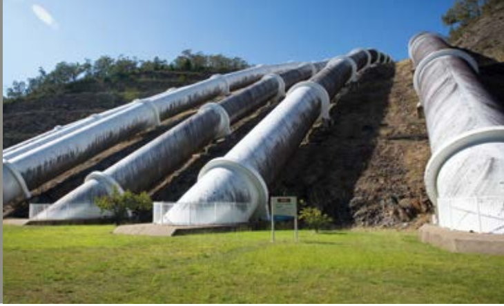
Water pipes in the Snowy Mountains, Australia. Source: Shutterstock
