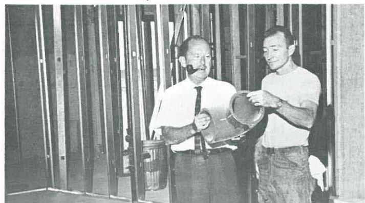
Construction of facilities for the Germfree Life Research Center on the third floor of the Parker Physical Sciences Center is inspected by Dr. Joel Warren, left, and electrical foreman Robert Smith. Dr. Warren is director of the Center.
