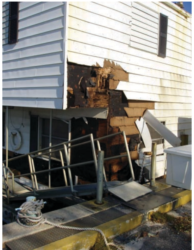
This is some of the damage to the houseboat.
